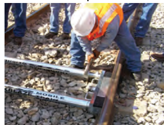
Inserting the MTW into the track and expanding the system via the threaded support poles
